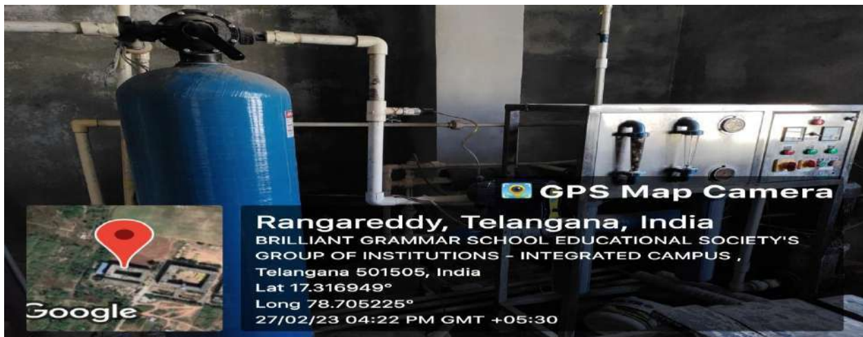
RO water plant.
